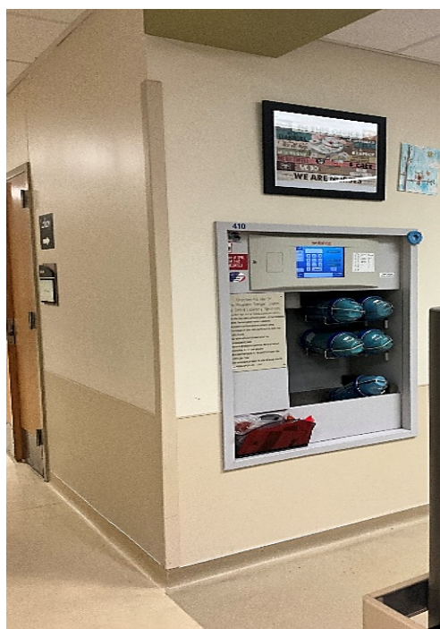
Figure C.2. Unsecured tube station area.
