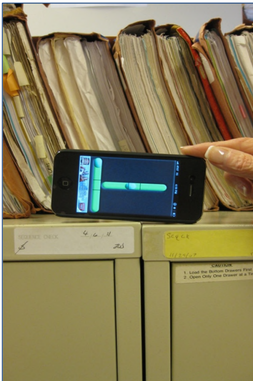
Figure 4 – Sloping floors cause cabinets to shift due to the increased weight over time
