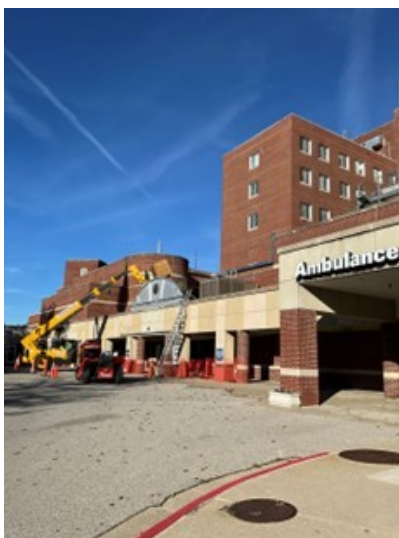
Figure C.3. Unattended construction site at clinic entrance.
